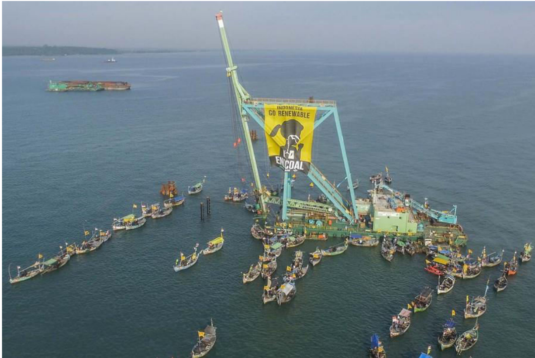
Activists occupy a piling barge off the shores of Bantang, Central Java, on Thursday (30/03) to call for the termination of a coal-fired power plant development project in the area, known as the Central Java Power Plant. (Greenpeace Photo/Ulet Ifansasti)
